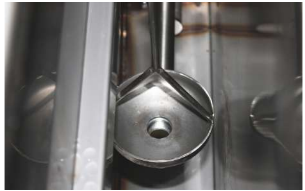
Interior detail of auxiliary tank.
